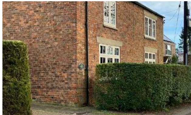
Figure 78: Red brick on a historic cottage.
