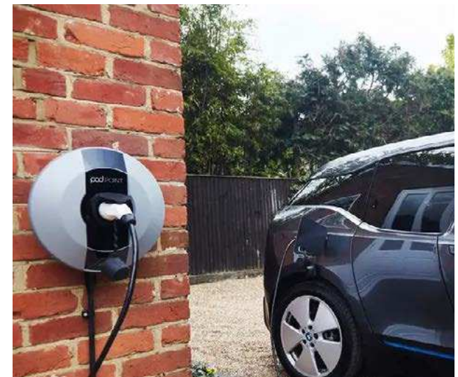
Figure 119: Home electric vehicle charging point located at the side of the dwelling to minimise the visual impact.
